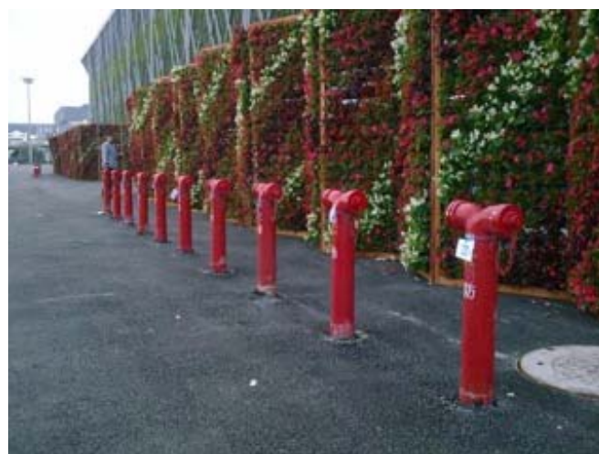
Fire hydrants at the ready outside the Expo site
